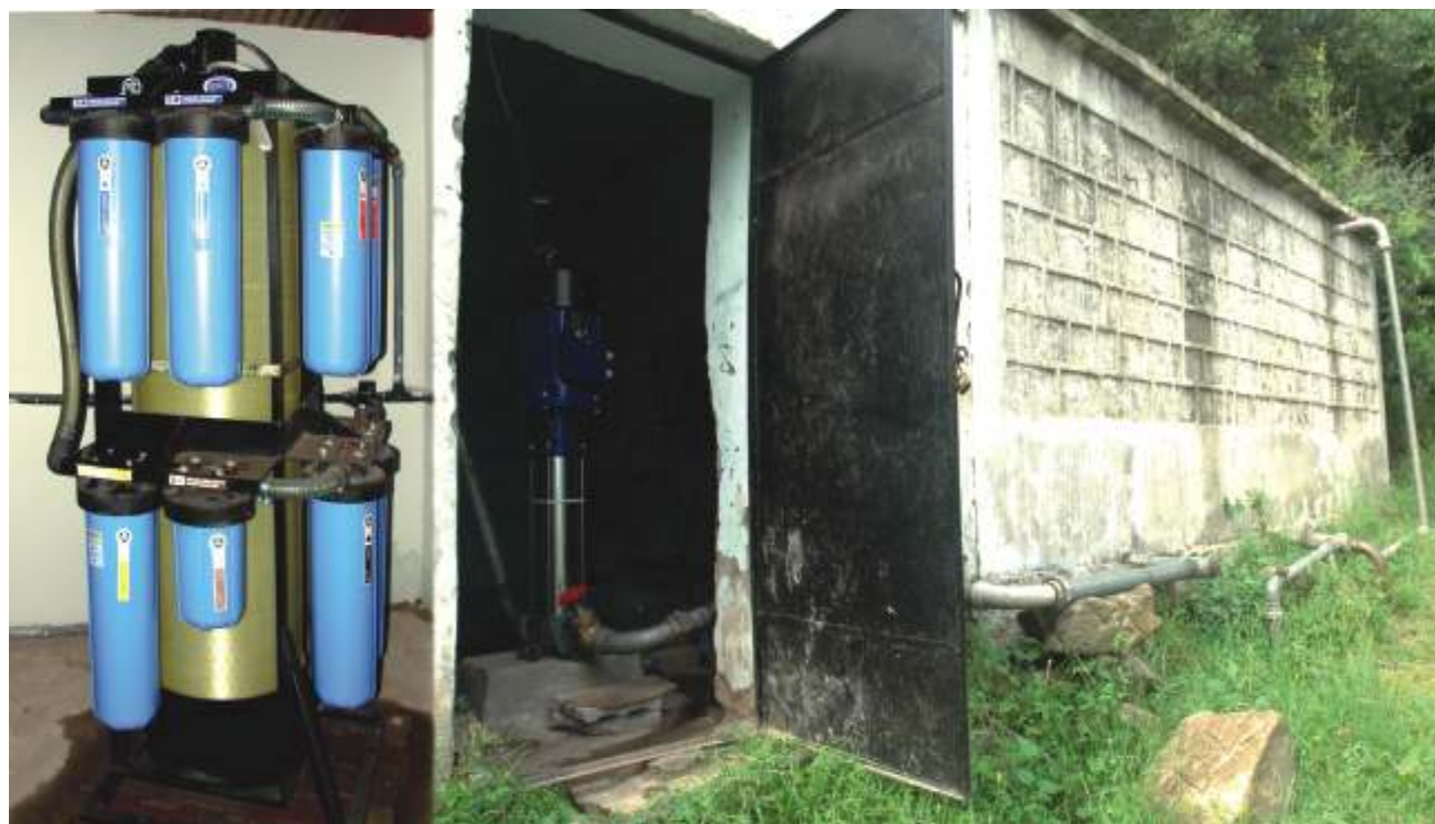
Water Filtration Plant with Ground Water Pumping Scheme
