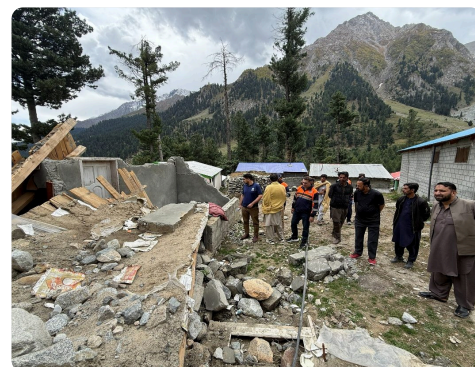
Damaged structures — Naltar Bala
