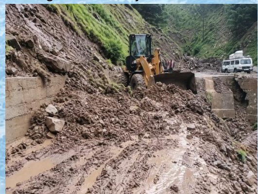
Figure 22: Slope instability causing road embankment failure and landslide damage during heavy monsoon rainfall.
