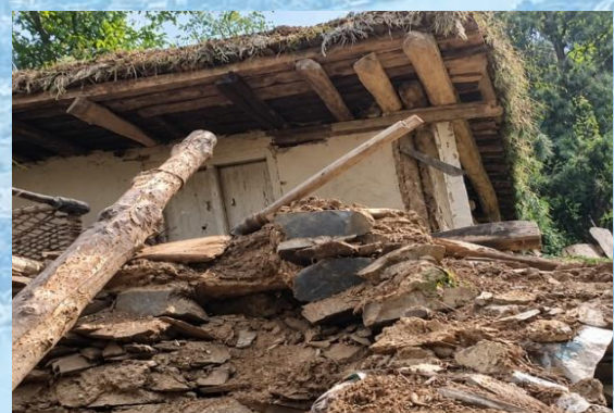
Figure 16: Soil settlement causing foundation displacement, severe wall cracking, and partial structural collapse during monsoon flooding.
