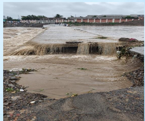
Figure 21: Undersized and debris-choked culvert causing overtopping, road inundation, and embankment erosion
