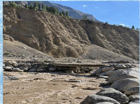
Figure 25: Aging bridge infrastructure showing severe deterioration and vulnerability to monsoon flood flows.
