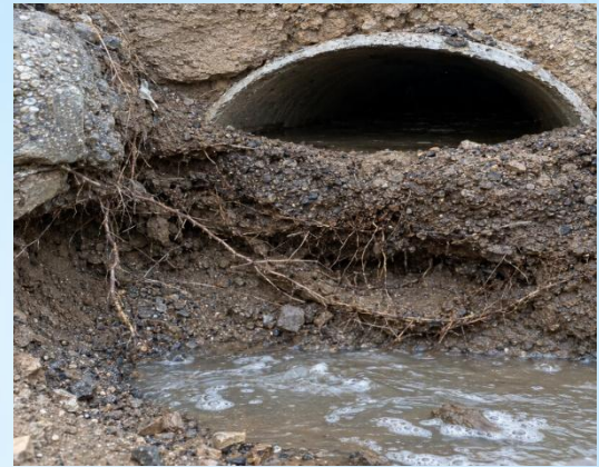
Figure 23: Sediment and debris accumulation clogging culvert openings and obstructing floodwater flow.
