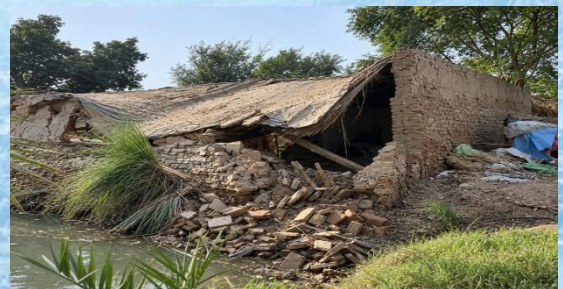
Figure 19: Foundation failure and severe structural cracking caused by prolonged waterlogging and soil instability.
