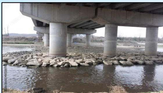
Figure 61: Hydraulic conveyance structure designed for flash-flood discharge conditions.
