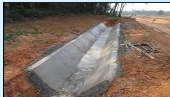
Figure 62: Trapezoidal drain channel providing efficient conveyance of concentrated runoff.
