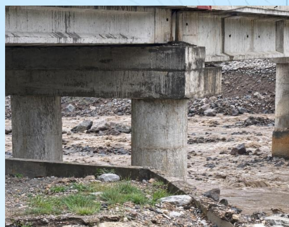
Figure 26: Bridge foundation Vulnerability due to unregulated sand & gravel mining
