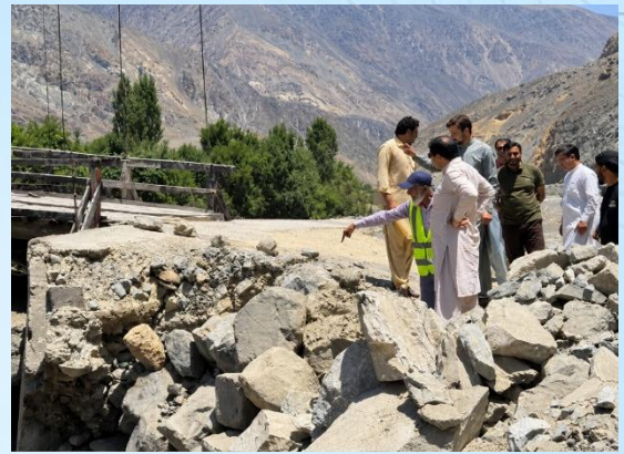
Figure 20: Bridge failure and structural distress under high-velocity flood flows.
