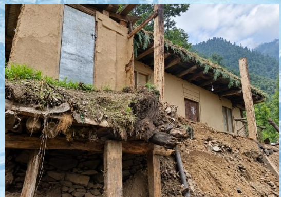
Figure 13: Ground movement and differential settlement causing severe cracking, tilting, and partial collapse of a hillside residential structure.
