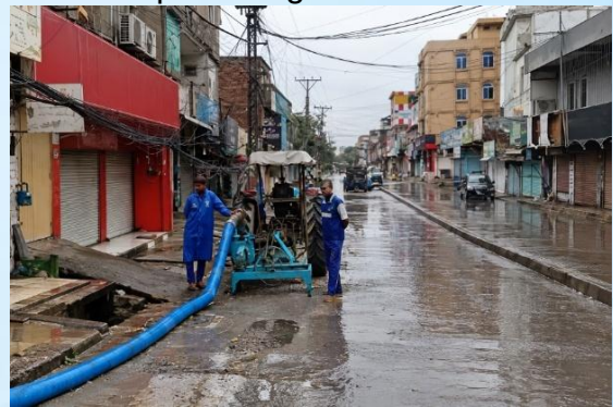
Figure 18: Inadequate drainage planning causing prolonged waterlogging around residential structures during monsoon rainfall.
