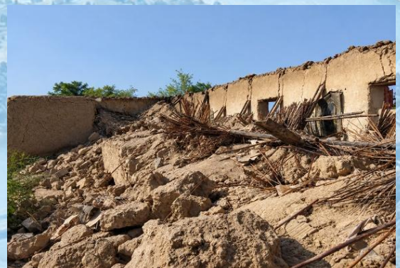
Figure 10: Flood Affecting Residential Structures (Inadequate Foundation Design)
