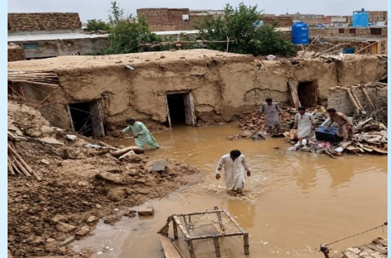
Figure 11: Foundation soil erosion and scouring causing structural instability during monsoon flooding.
