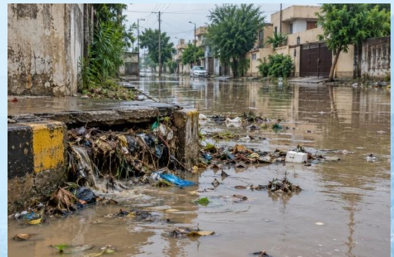
Figure 12: Blocked drainage causing severe urban waterlogging during monsoon rainfall.
