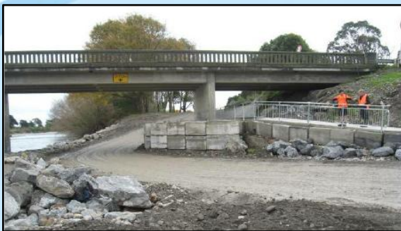
Figure 59: Concrete block protection installed around a bridge pier foundation.
