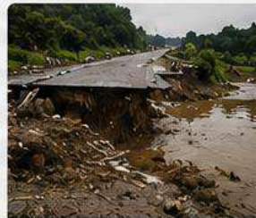
Road & Access Damage
