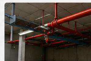
Sprinkler Systems & Fire Suppression
