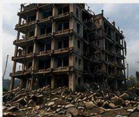
High-Rise Building Damage
