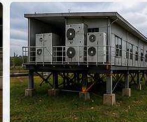
Elevated Utilities & Critical Systems
