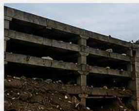
Parking Structure Collapse
