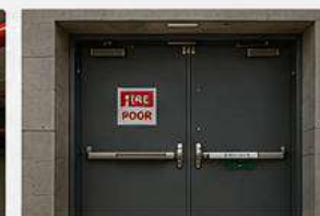
Fire-Rated Doors & Compartments
